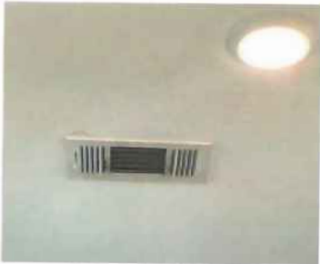
Water Stains - Kitchen & Living Room Vent
