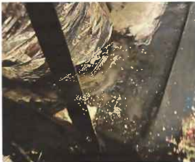
Typical Conditions - HVAC System
