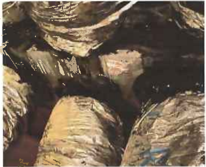
Typical Conditions - HVAC System
