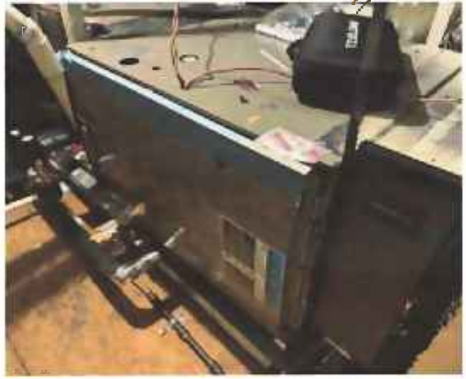
Typical Conditions - HVAC System
