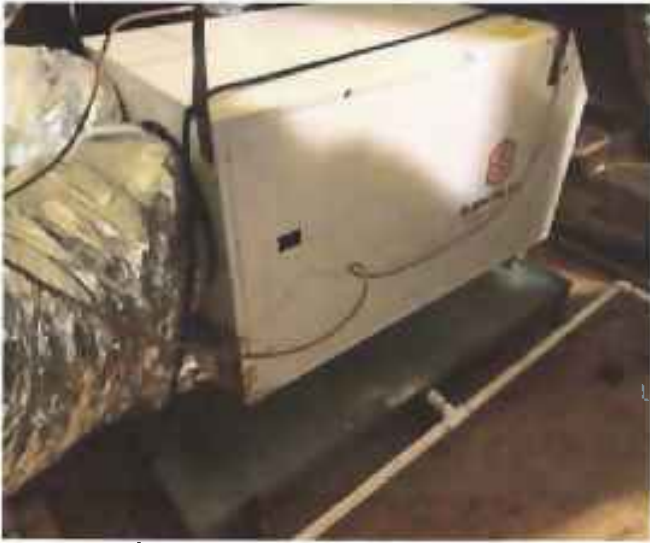
Typical Conditions - Dehumidifier
