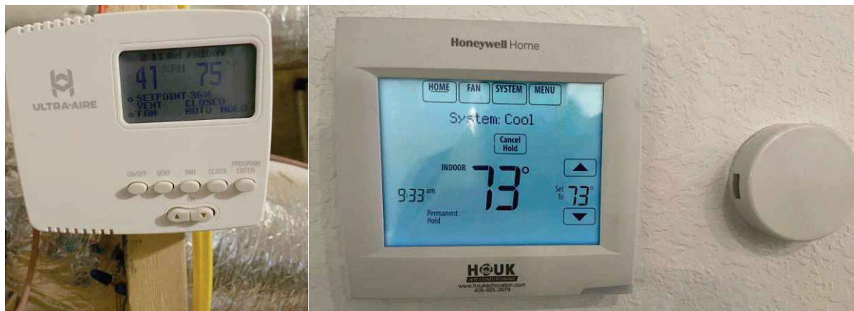
Figure 1: On the left: the attic-mounted DEH3000R humidistat; on the right, the thermostat and humidity sensor. The round humidity sensor is wired directly to the DEH3000R controller.
