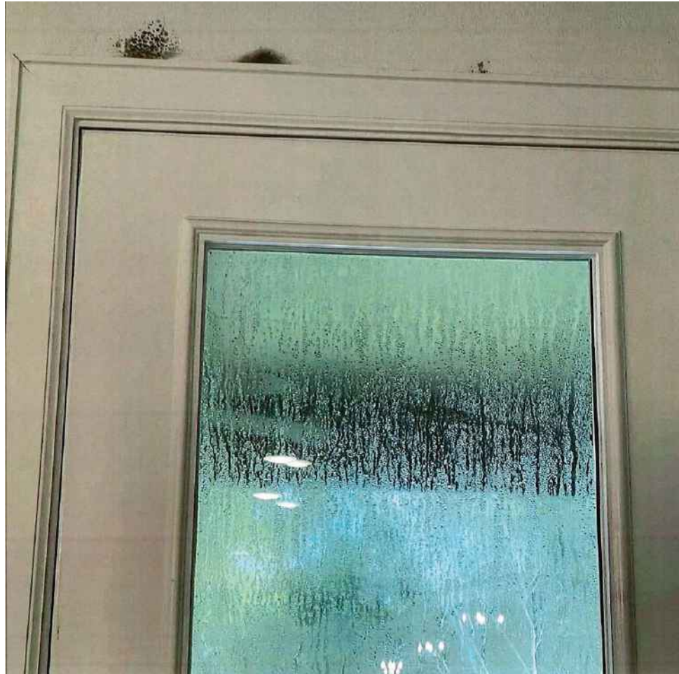
Figure 11 Note the lack of distortion in the reflections of the interior lights on this door's window; this indicates that the condensation is outside, not inside, the home.
