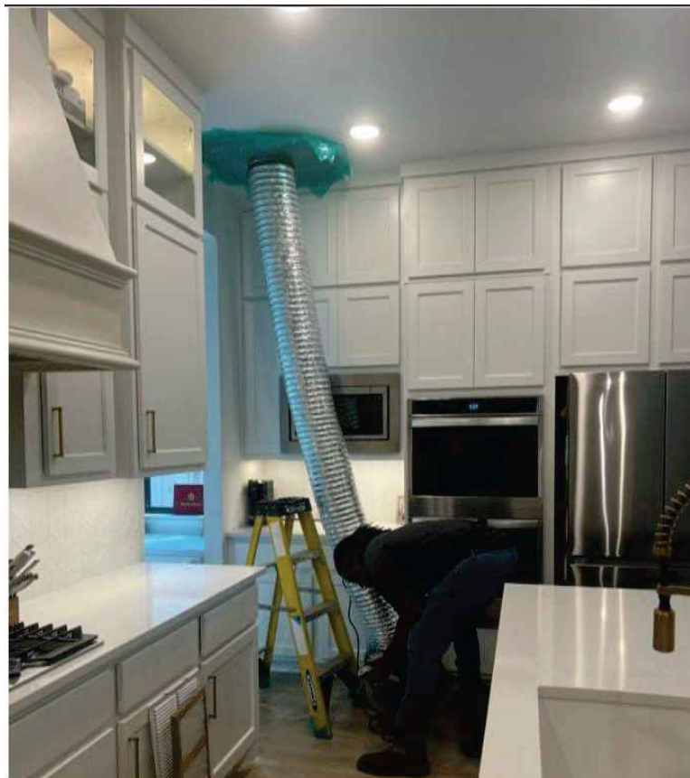
Figure 15: This photograph from the Apollo BBC report appears to show a duct pressurization test being performed. However, the connection is to an outdoor vent, not to a return duct of the HVAC system.
